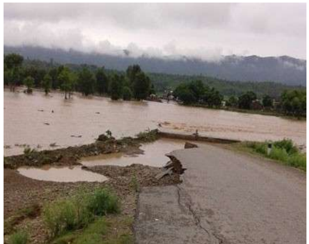
Road damaged by flood
