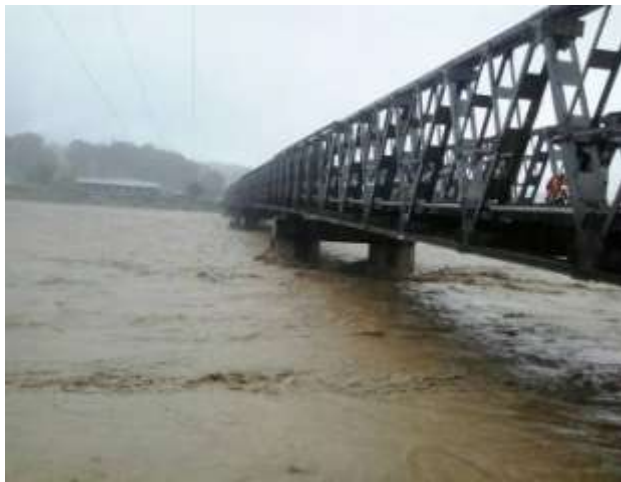
Chitwan - Nawalparasi Bridge in risk
